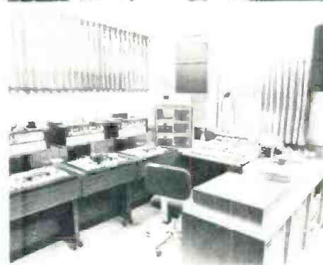
Each of the five production studios is equipped with a McCurdy SS8600 console, Technics SP 10 MKII turntables, ITC Series 99 cart machines, Onkyo cassette deck, MCI JH 110B reel-to-reel tape decks, Crown D300 monitor amplifier, Crown D60 headphone amplifier, and Beyer M-500 mics
